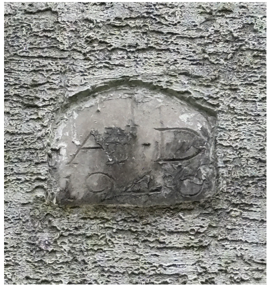
Fig. 12. The date stone as it currently appears, surrounded by stucco on mesh that was added much later and is beginning to fall away. Current photo.
