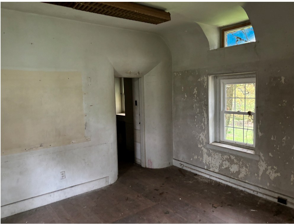
Fig. 33. Curved edges around the doorway upstairs in the c. 1810 portion of the house.. Current photo.
