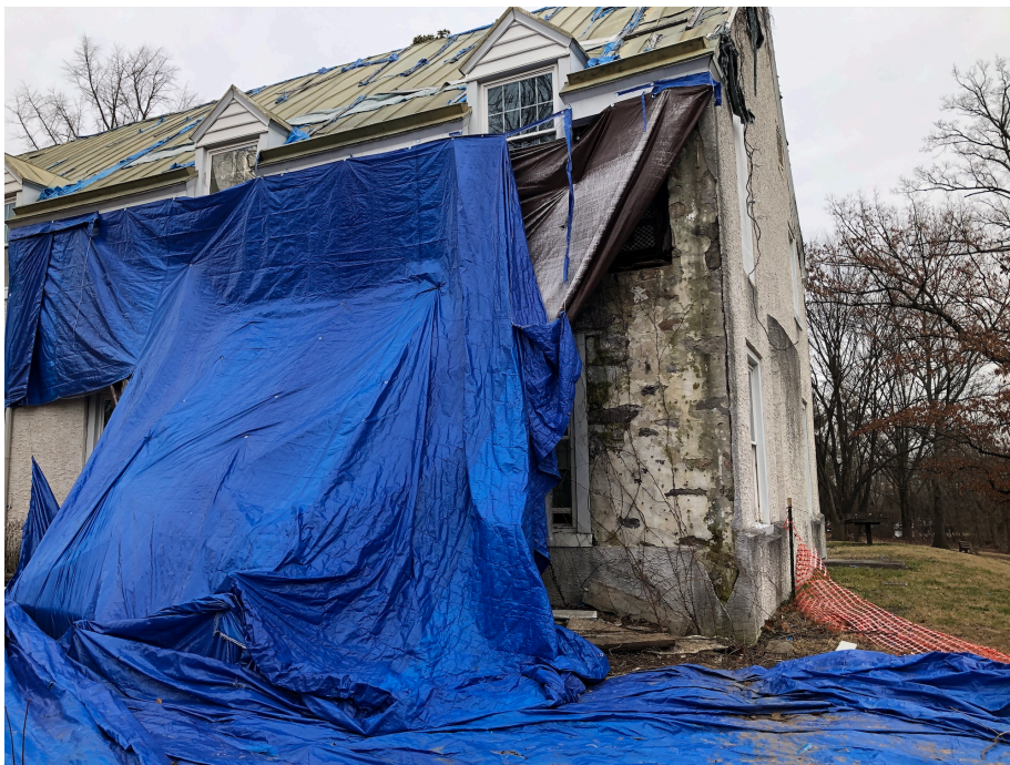
Fig. 8. The southwest corner of the 1932 Okie addition showing the falling away of the stucco on mesh, revealing the intact original stucco on stone. Current photo.
