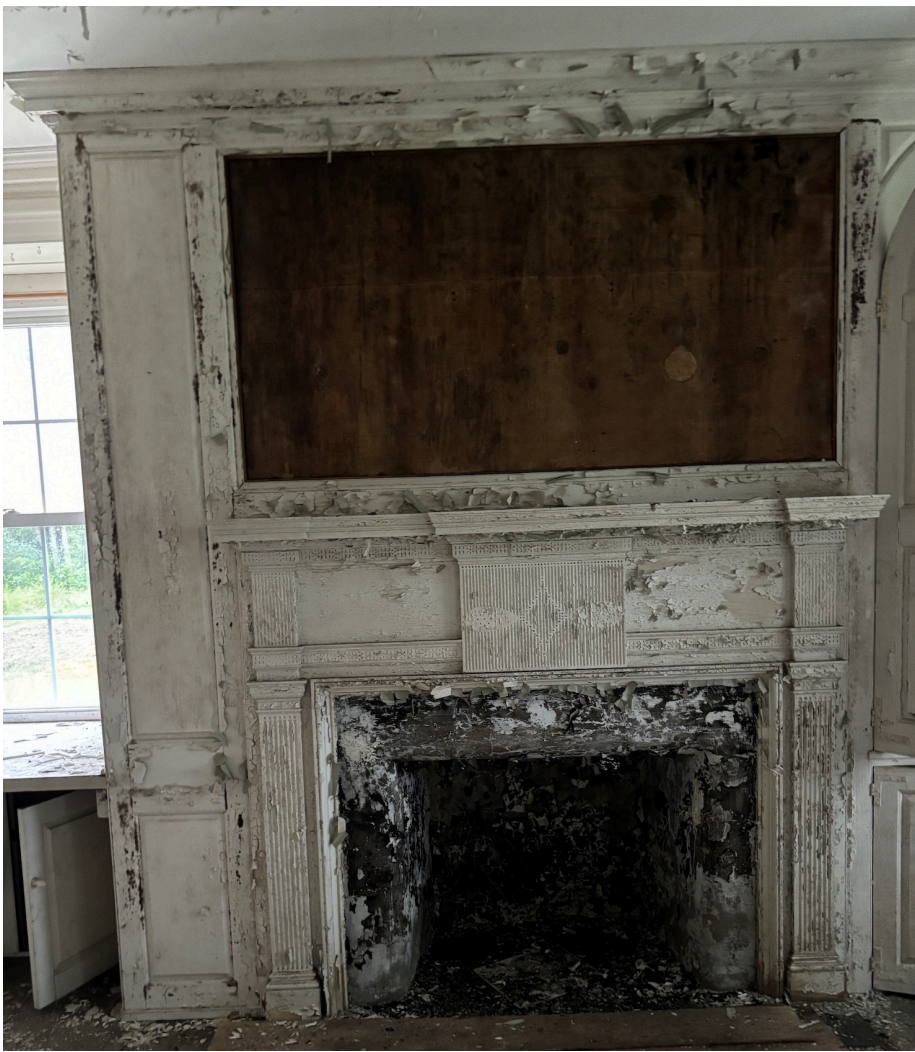
Fig. 16. Fireplace at the west end of the c. 1820 portion of the house with the carving shown in the plans below. Current photo.
