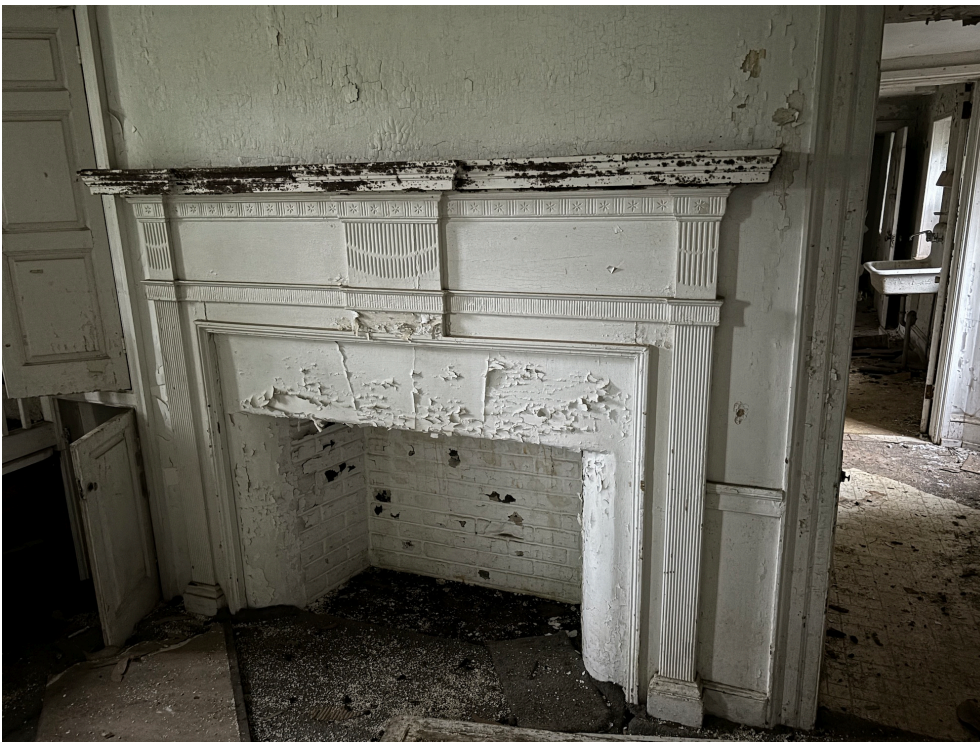
Fig. 16. Fireplace at the east end of the c. 1820 portion of the house. Current photo.
