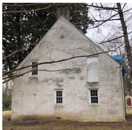
Fig. 46. The east side of the house, showing the emergency exit from the servants quarters second floor. Current photo.
