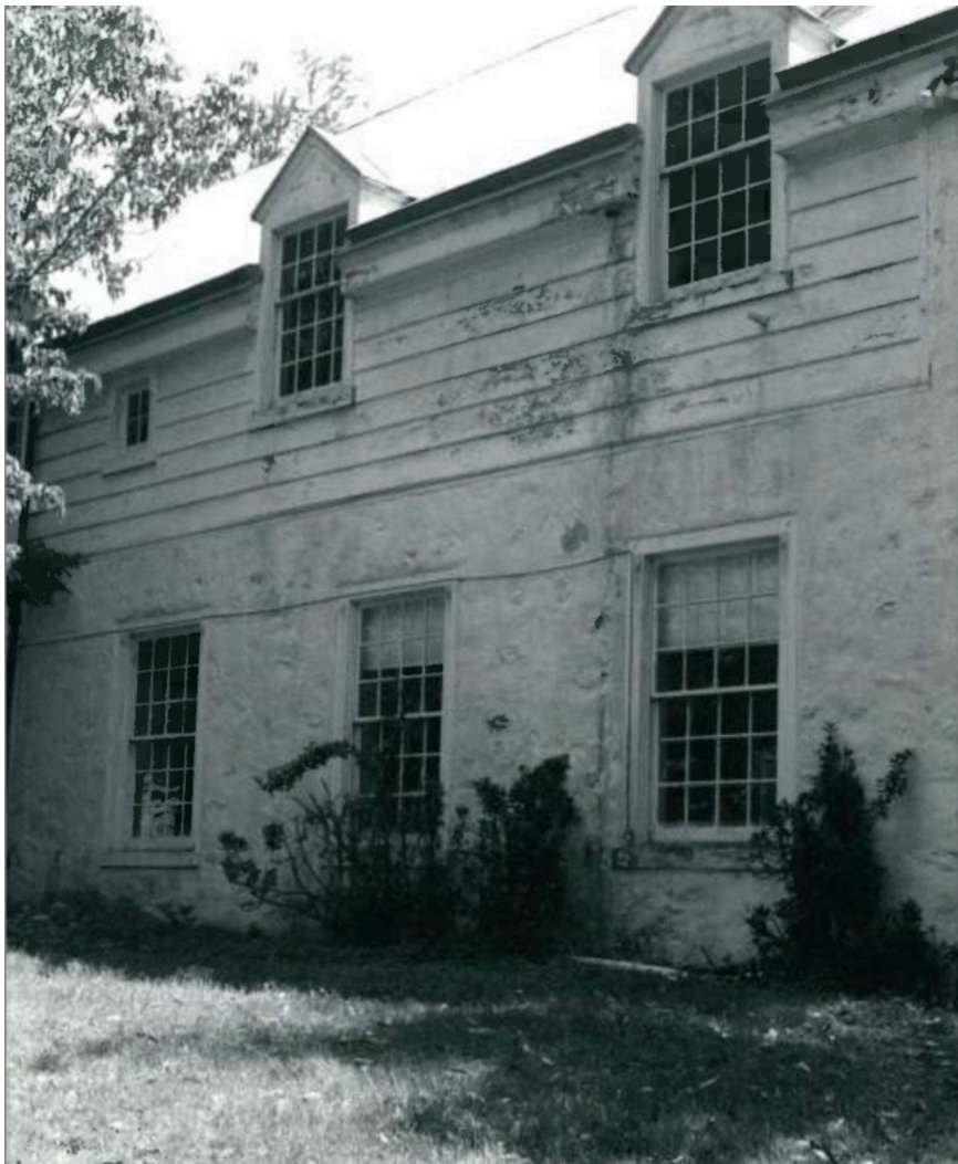
Fig. 14. The west side of the 1932 addition showing the dormer windows that break the roofline. Photo by Dave Broida in 1979.
