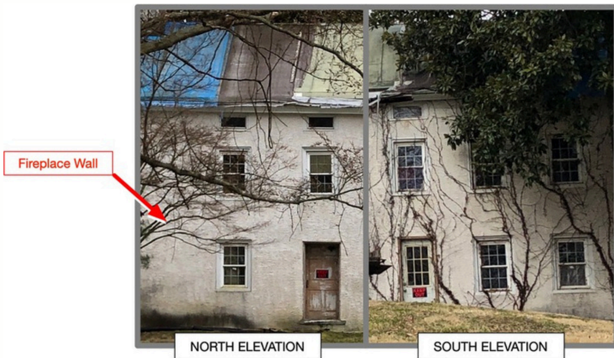
Fig. 13. North and south elevations of the 1810 portion of the house. The north face of the section does not match the south face. The asymmetry consists of a large blank space where the fireplace wall is.
