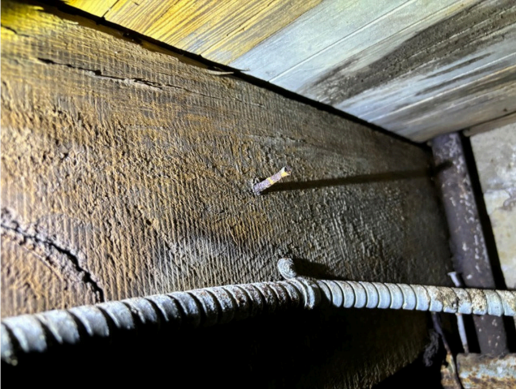
Fig 9. Joists in the basement of the Moore-Irwin House. King of Prussia Historical Society.
